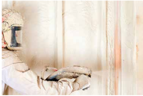
The spray foam retrofit provided benefits in terms of effective air sealing and ease of application. However, the installation of this scenario disrupted the building activity because the space required vacating during installation as well as for a specific period after installation.
